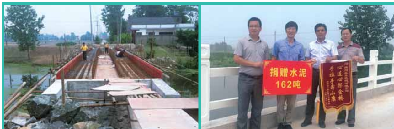
The construction and completion of a bridge with the aid of Yangzhou Ya Dong in Fanchuan Town, Jiangdou District of Yangzhou City
